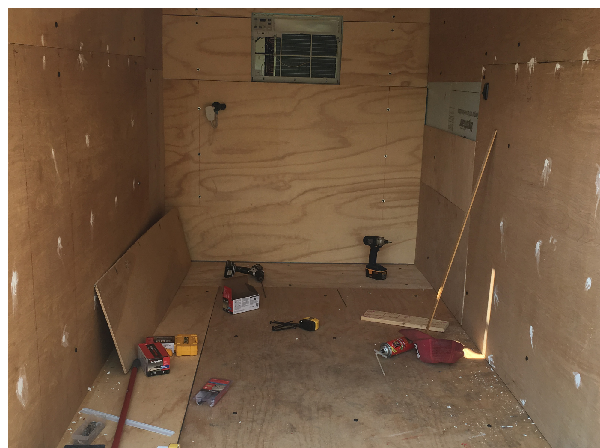
We covered all of the foam board with new and recycled plywood. (Most of the walls are the original paneling; the floor and ceiling are new.) If you want to learn from our mistakes, pick the right hardware and, for the love of all that's holy, mark your studs every step of the way!
