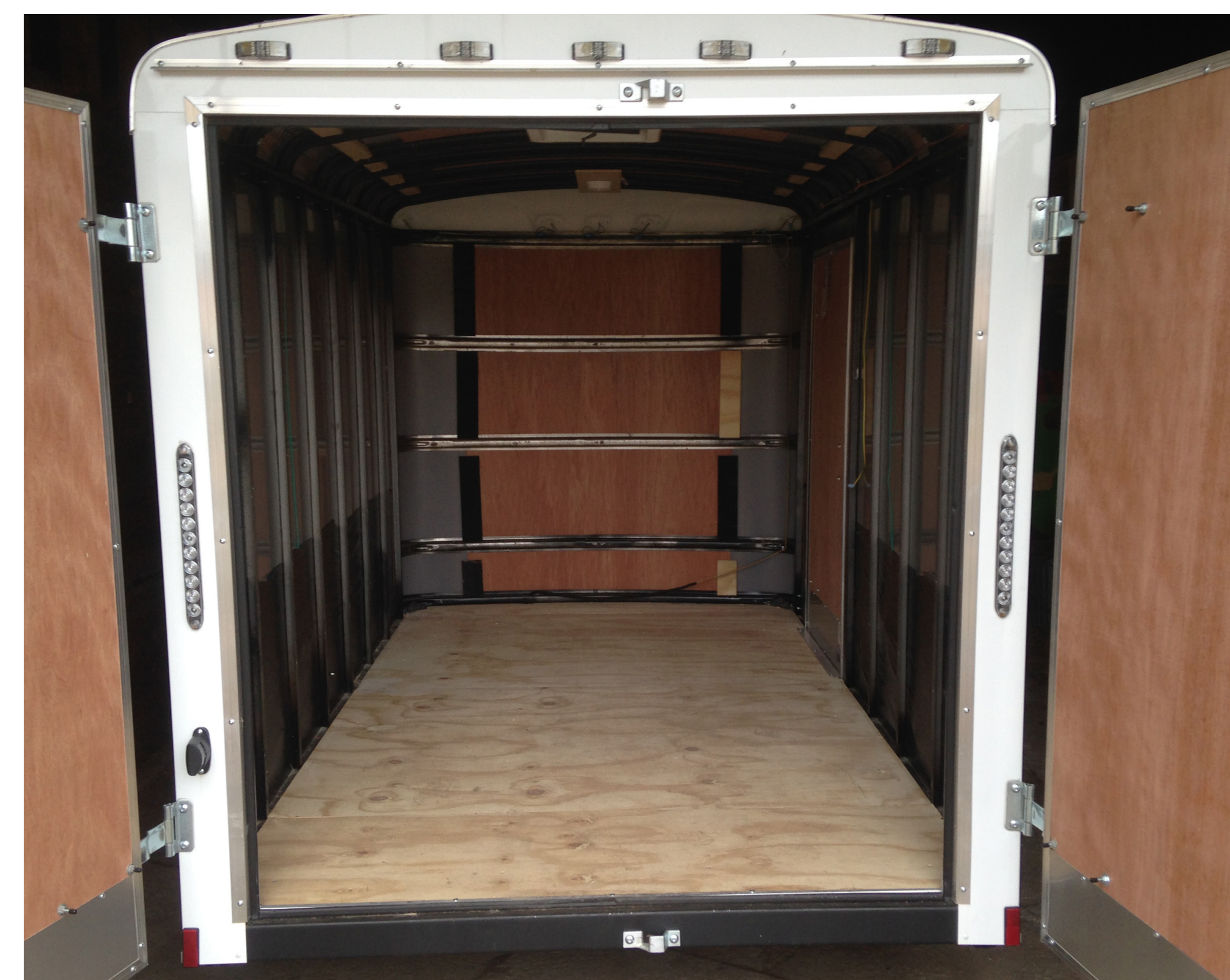
Trailer with all the plywood removed and electrical wiring and lights taped up. Next, we made a hole for the AC unit in the back and then measured, cut, and framed out the foam board insulation.
