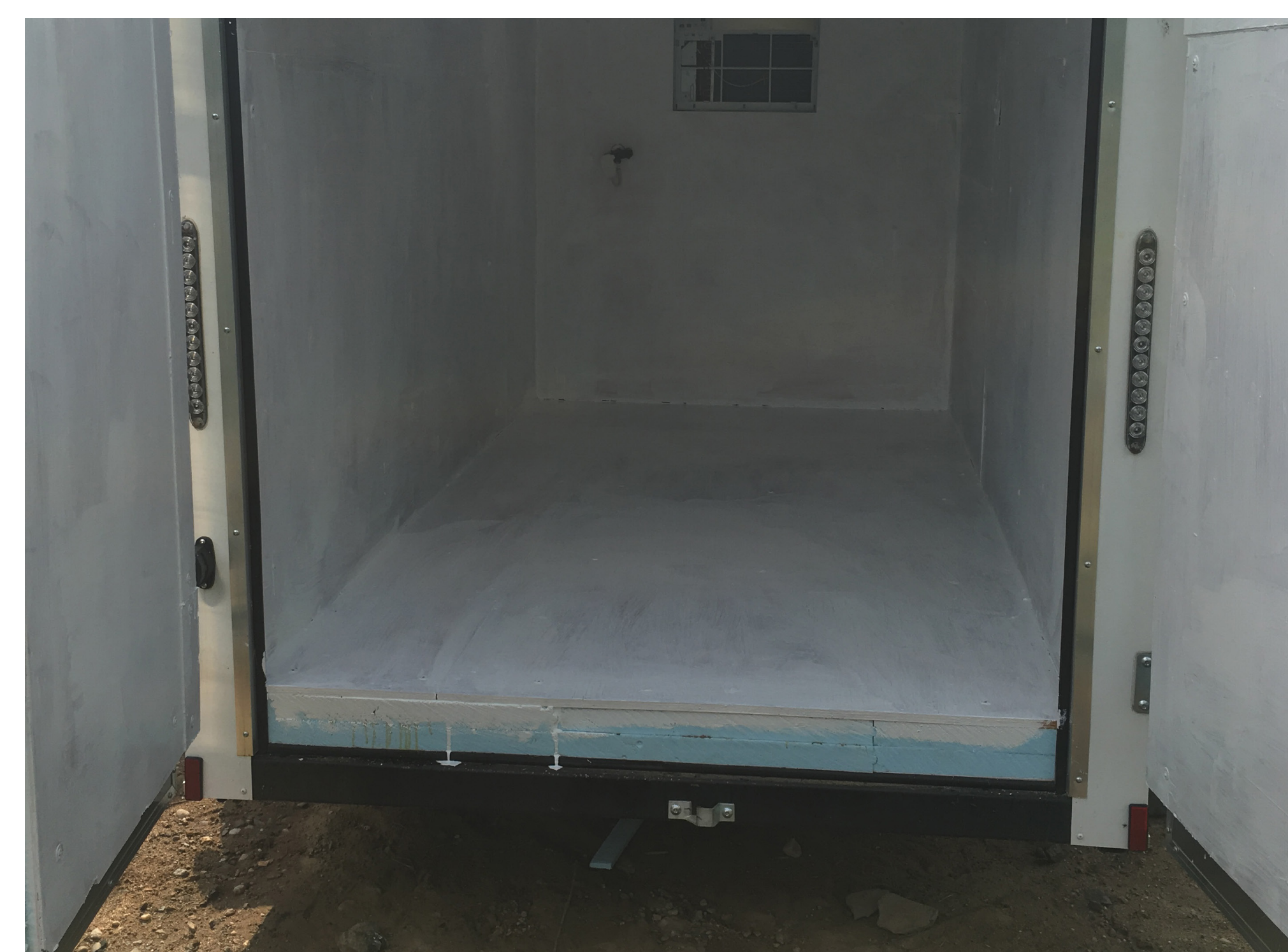
After you've filled all the gaps with putty and spray foam, don't forget that this beast is going to be full of freshly washed vegetables! Put some paint on it. Mildew-resistant bathroom paint will work after you've applied a healthy lathering of polyurethane.
